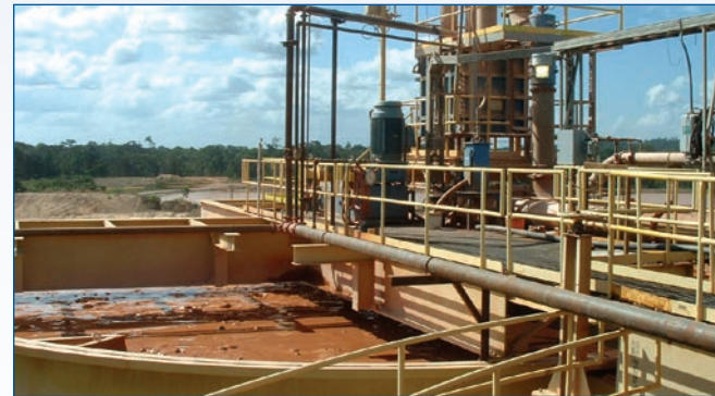
200 HP, LHX-160 mixers on 52.5' diameter gold leach tank.
