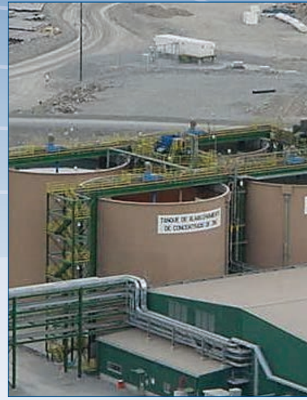
LHX-160 with 150 HP drives operating on zinc and copper concentrate tanks.
