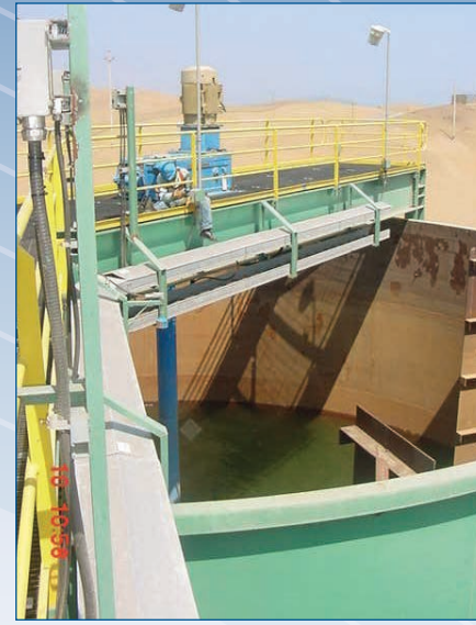
LHX-150 maintaining solids in suspension on a 49' diameter storage tank.
